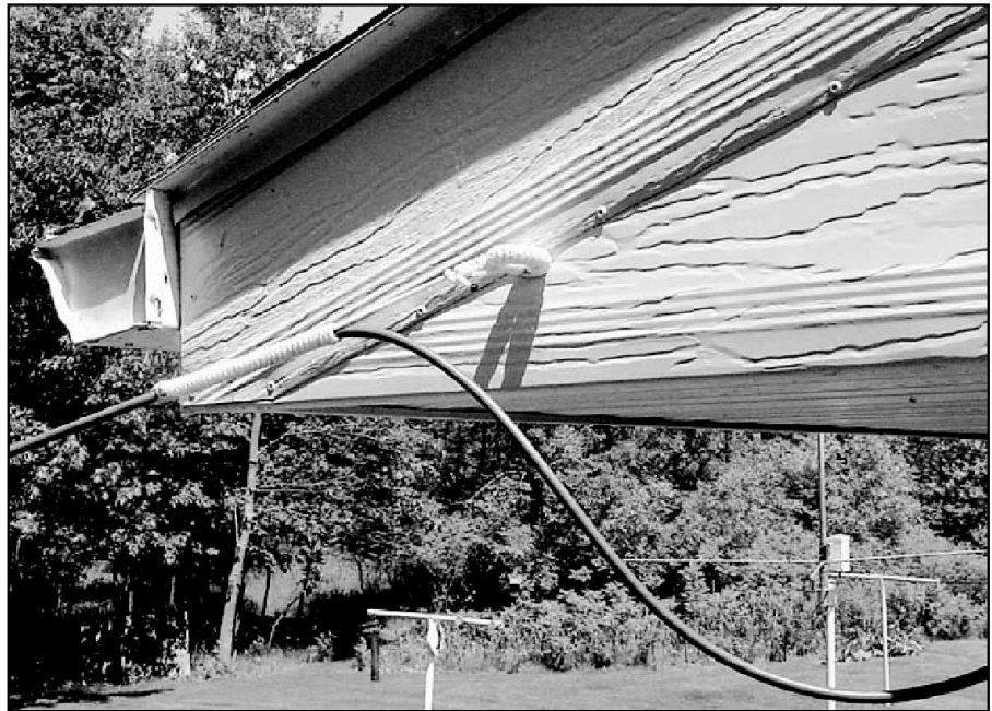
Figure 1 — RG-8X coax anchored to the author's house.
