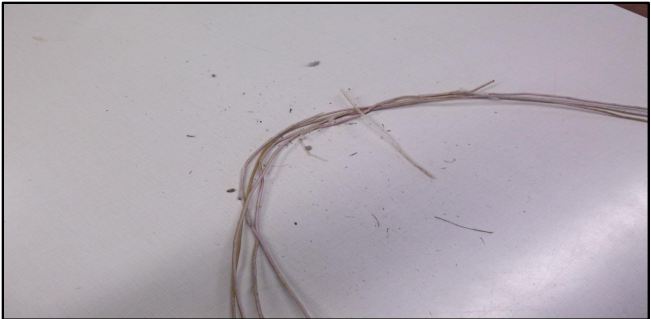
Figure 1 - Sample of degraded #12 radial wire.
