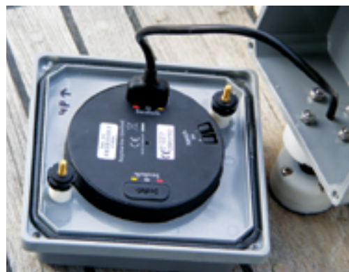
The foam gasket around the cover ensures that the junction box is waterproof.
