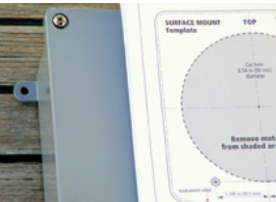
Using the template that came with the control head, Rich cut the hole and drilled for the fasteners.
